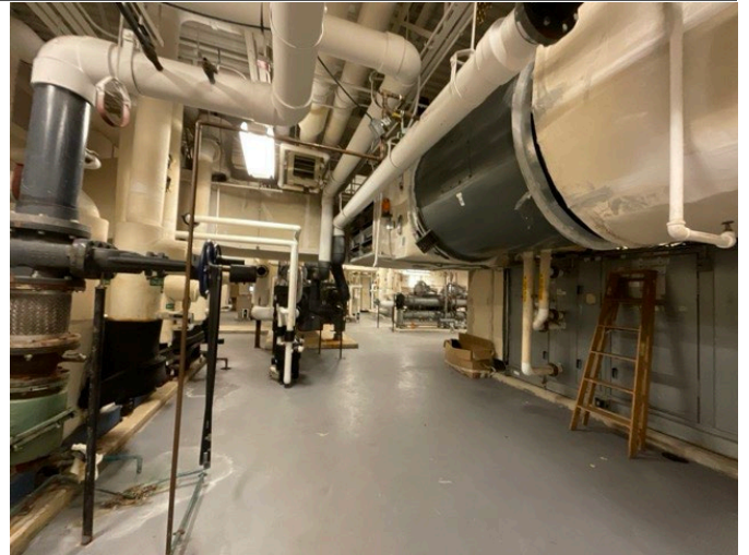
8 - MECHANICAL PENTHOUSE ROOM
