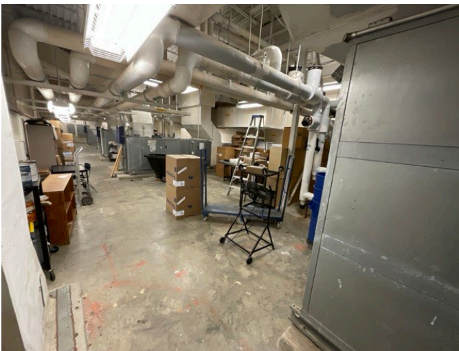
9 - MECHANICAL PENTHOUSE ROOM
